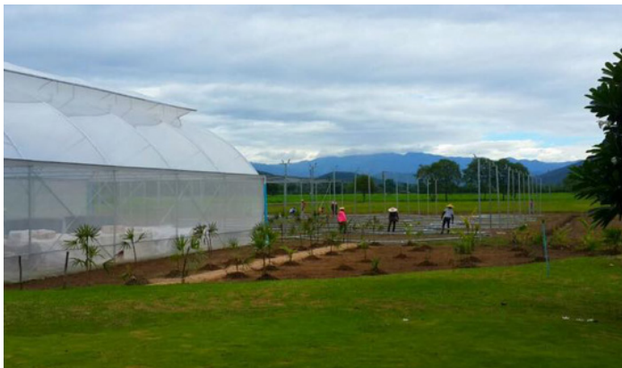
Workers setting up a greenhouse where an aquaponics systems will be housed
